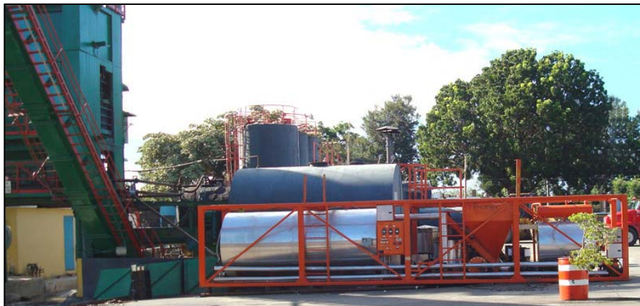
Phoenix Industries' Asphalt Rubber blending plant operating at R & F Asphalt Unlimited's hot plant site in Coto Laurel, Puerto Rico
